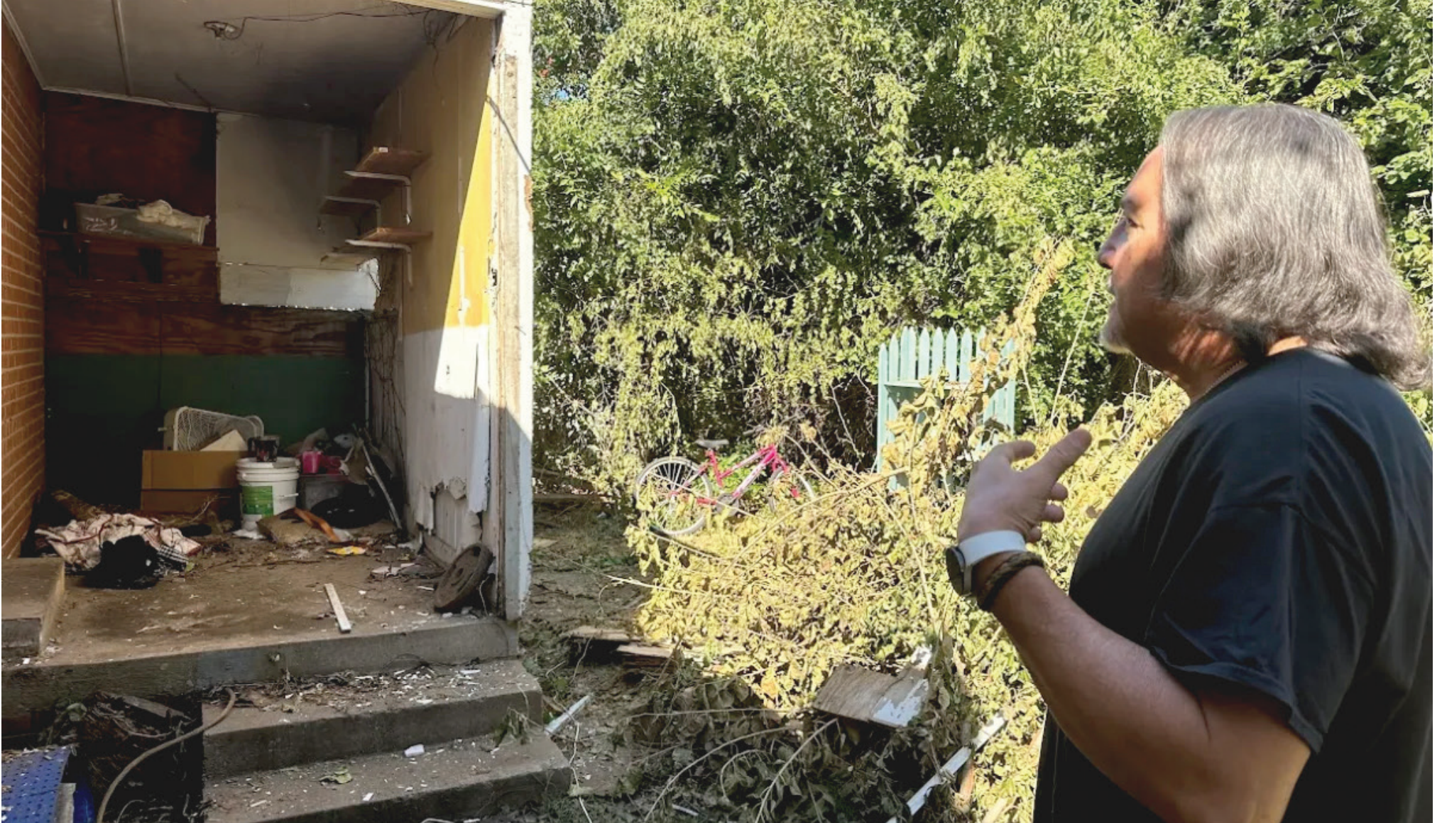
Harold Morris discusses the conditions of his falling-apart rental home owned by landlord Virginia Oldham. Oldham evicted Morris after he reported the home's problems to Oklahoma City Code Enforcement.
