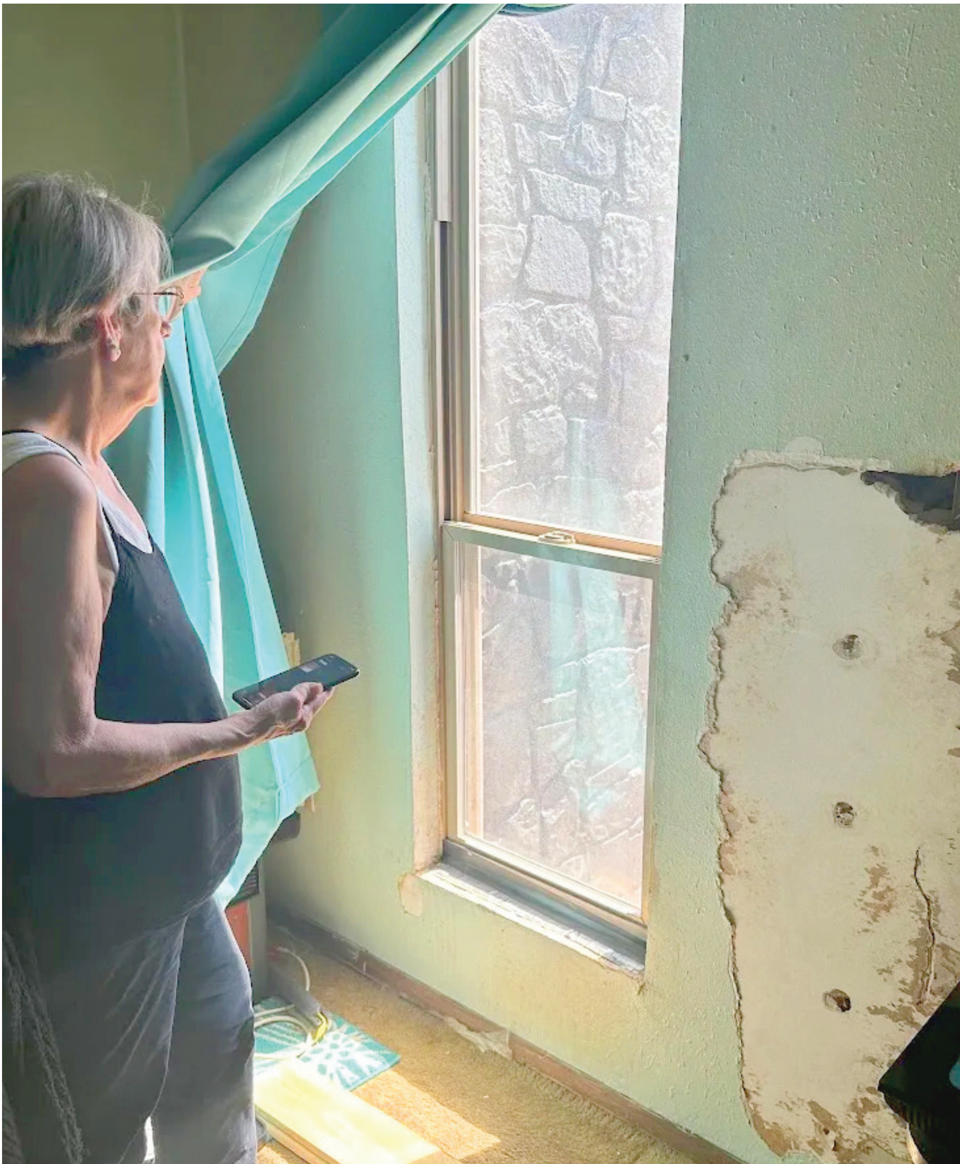
Shanon Van Gordon looks out a window in an unusable upstairs bedroom where rainwater and snow pour in the unsealed windows and gaping holes in walls go unfixed.
