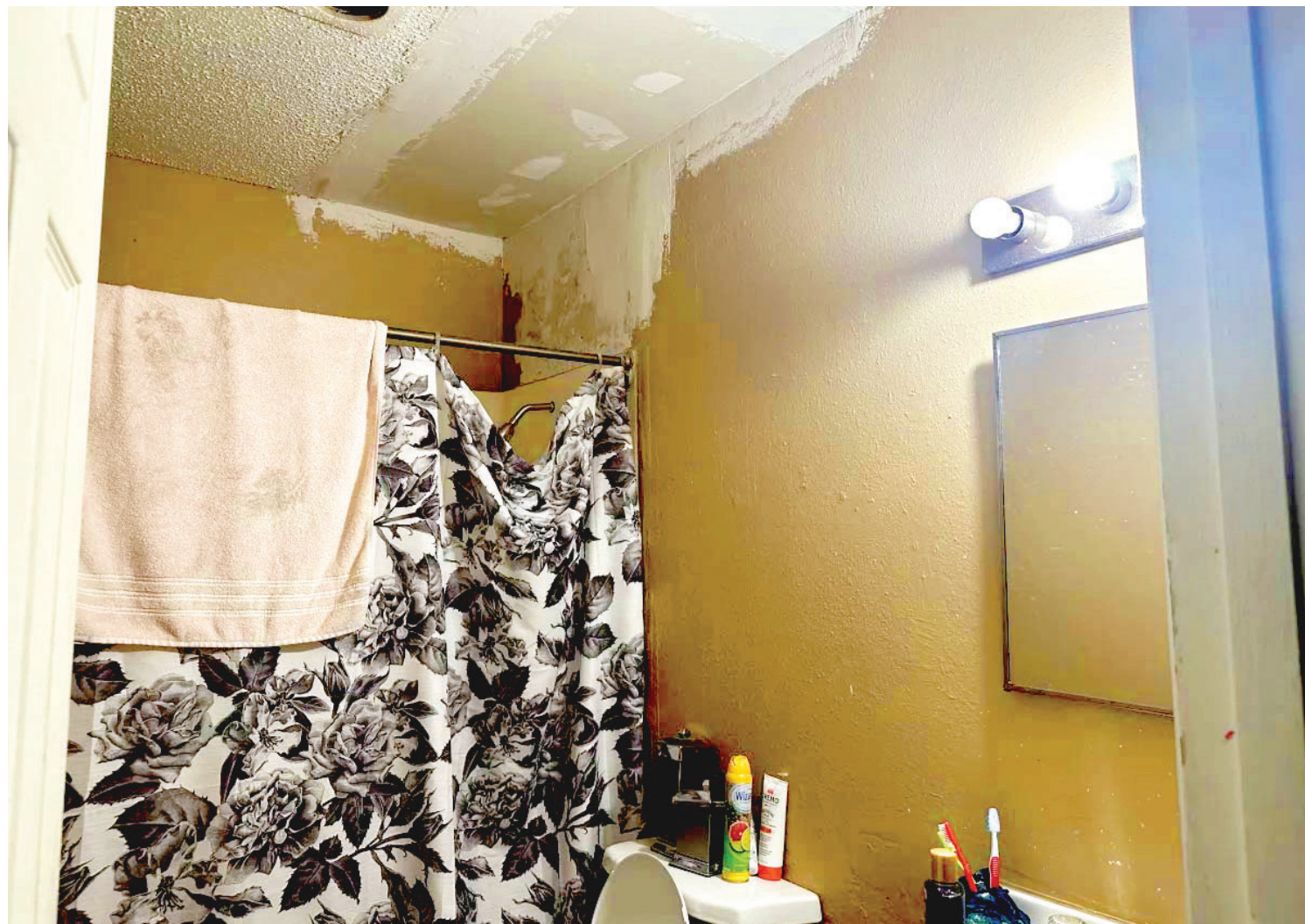
The ceiling in Georgia Guerrero's bathroom caved in and was patched by apartment maintenance staff at Elm Terrace Apartments in Duncan.
