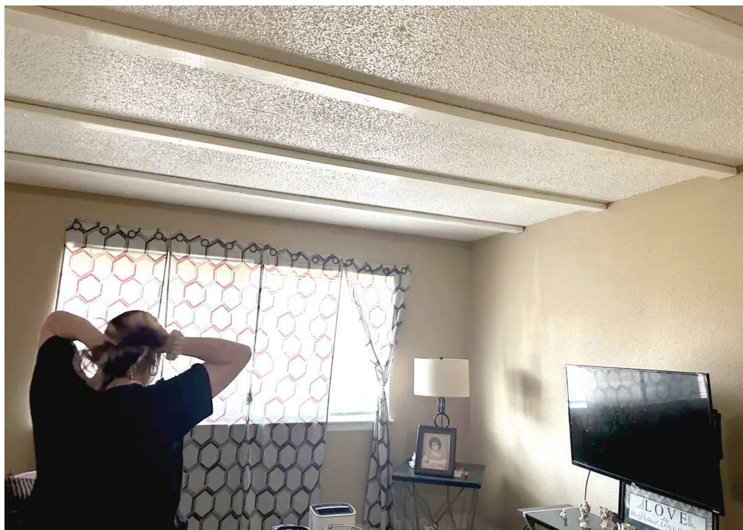
Georgia Guerrero shows the beams that have been installed on her ceiling to keep the upstairs from caving in at Elm Terrace Apartments in Duncan on Sept. 8, 2024.
