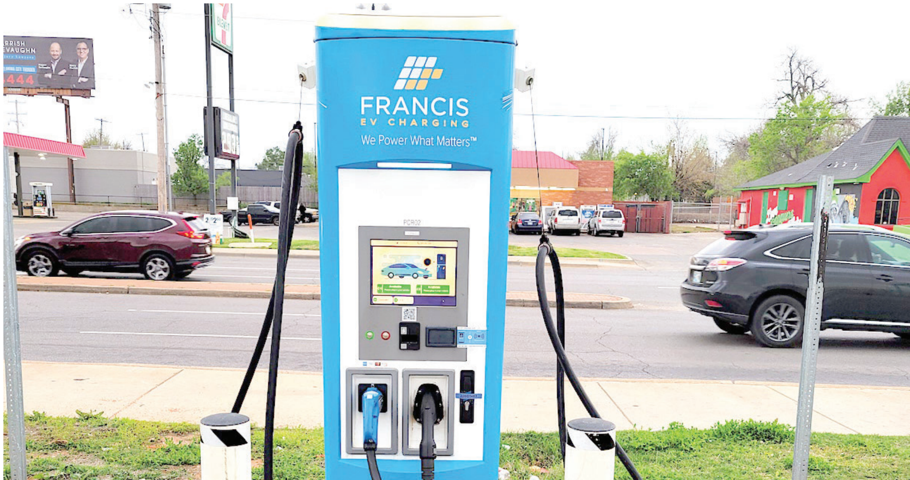
A FRANCIS ENERGY EV CHARGING STATION is located near the intersection of Northwest 23rd Street and North Pennsylvania Avenue in Oklahoma City. PHOTO MICHAEL MCNUTT
